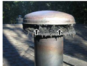
This chimney cap has a large amount of soot as well as creosote build-up and should be cleaned by a professional.
