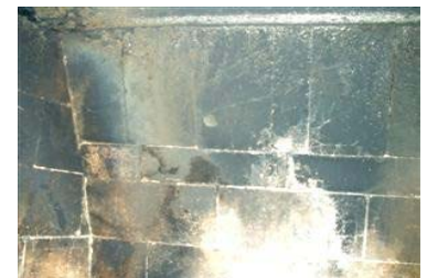
Tuck pointing is needed to prevent further deterioration.
